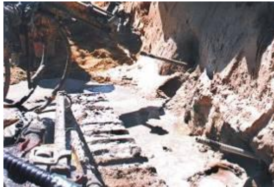
4. Soil nails installed into sand. Simultaneous drilling and grouting offers increased productivity and is beneficial to placement of the grout.
