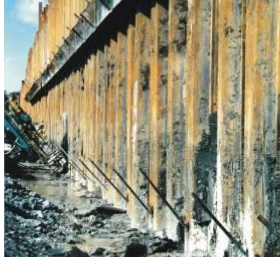
2. Temporary anchors for sheet pile tie back. Waling beams and anchors were installed at two levels, to provide increased support to the wall.
