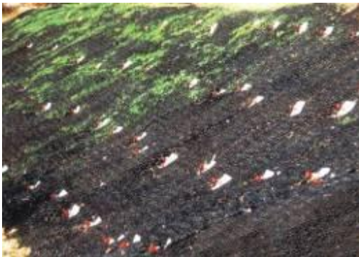
3. Galvanized soil nails securing an erosion control geomat, to resist soil slip. The grass on the slope was re-established by seeding the geomat.
