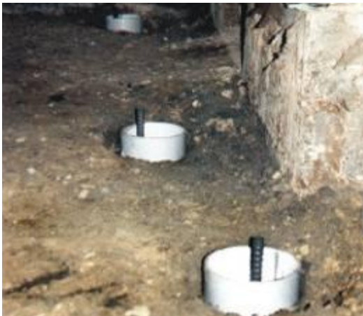
5. Underpinning of augered columns. The cast in situ columns was used to ensure lateral stability at the top of the micropile.
